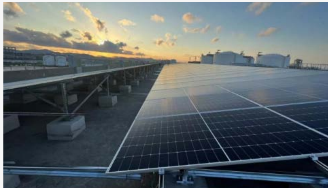
PV Sheds Built by Zhoushan Terminal
