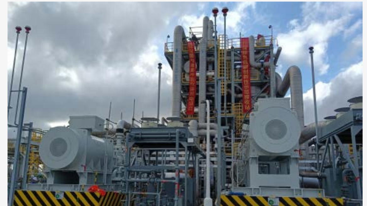
First LNG Dual-loop Cold Energy Power Generation Unit in China
